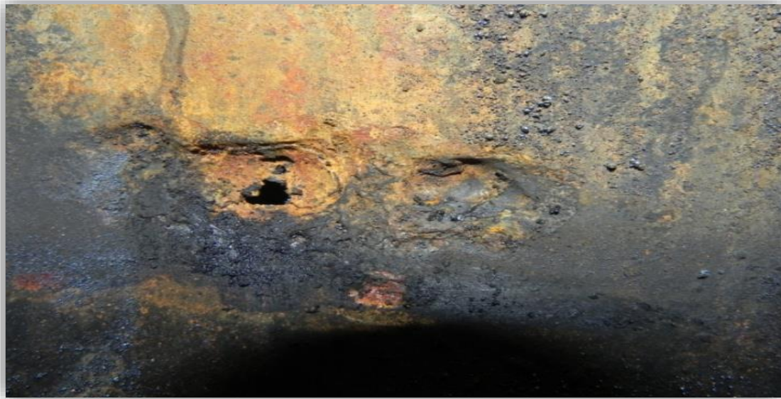
Figure 3.4. Confirmation of the Pipe having 6 Leaks with Defects up to 1” in Width
