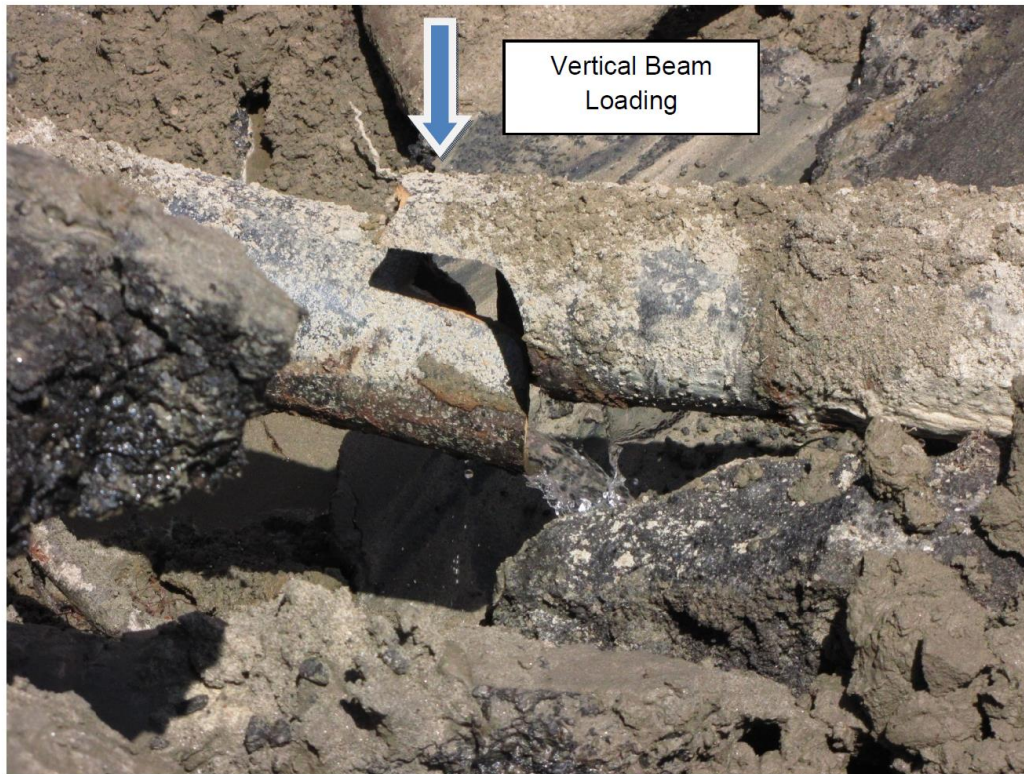
Figure 9.1. Vertical Loading and Loss of Pipe Support Leads to Circular or Circumferential Break in Cast Iron Pipe
