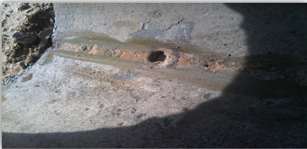
Figure 3.3. Confirmation of the Pipe having 6 Leaks with Defects up to 1" in Width
