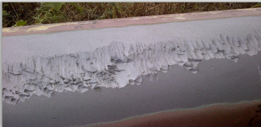
Figure 3.9. Pipeline Damaged due to a Paralleling Bore during the Reaming Stage
