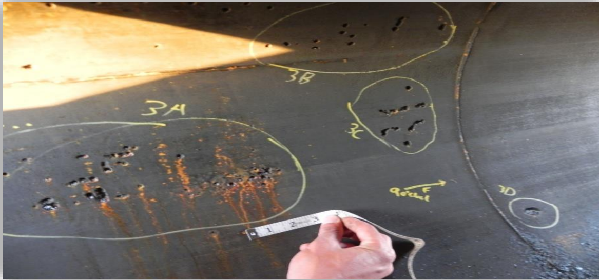
Figure 3.2. Results of the Tool Indicating 62% Wall Loss in Over a Hundred Different
