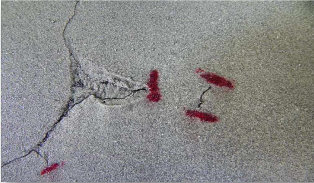
Figure 3.8. Example of Poor Pipeline Coating during Jeep Testing
