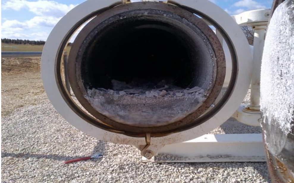
Figure 3.10. Formation of Hydrates Causing Ice Type Crystals to Form in the Pipeline
