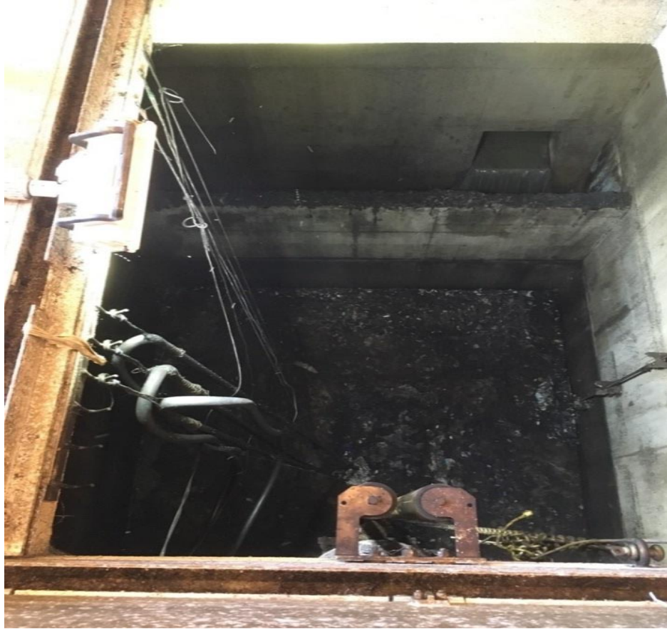
Figure 2.7 Inside View of Lift Station
