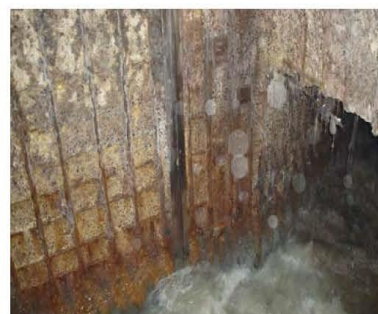
Figure 4 Reinforcing steel exposed after pressure washing
