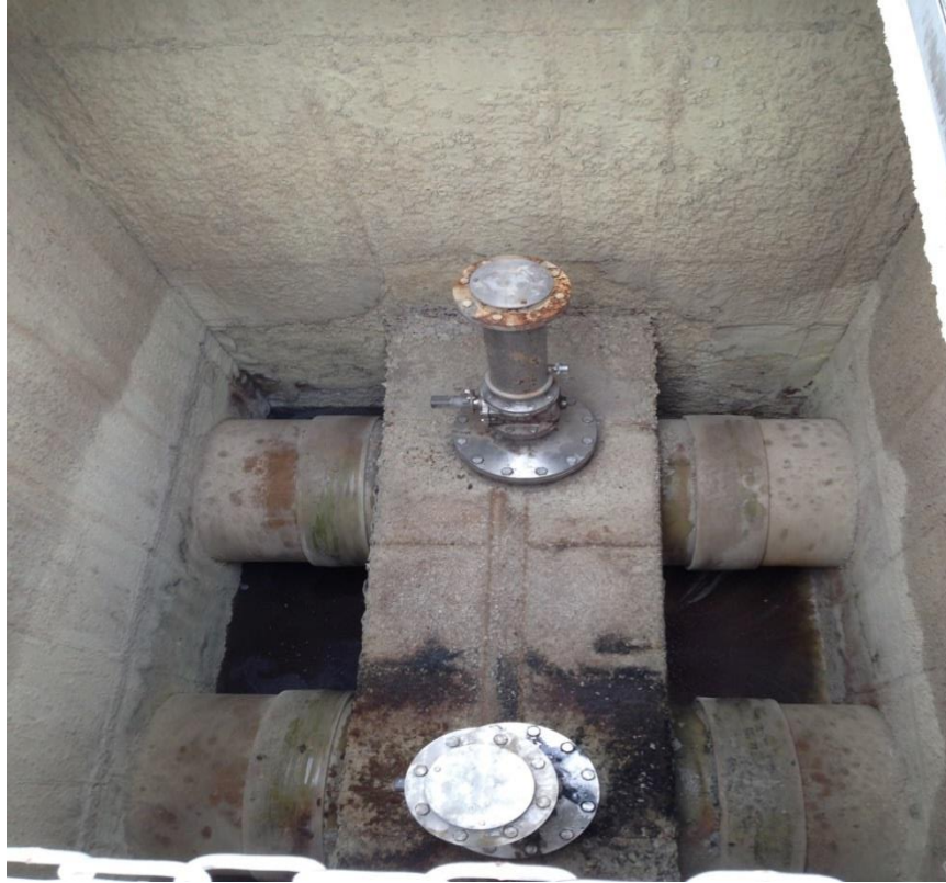
Figure 2.8 Concrete Valve Box after 9 Years of MIC
