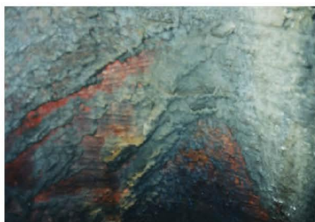
Figure 3 Corrosion prior to repair in 1999
