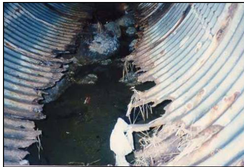
Figure 2.2 Deterioration due to Abrasion (Caltrans 2003)
