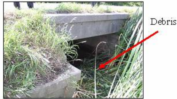
Figure 2.12 Debris at the Opening of the Culvert (Najafi et. al. 2008)
