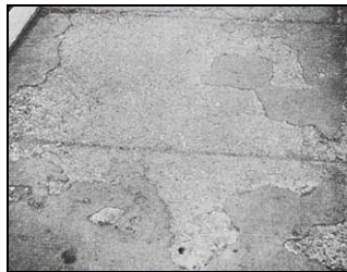
Figure 2.6 Scaling exposed on Concrete Surface.
