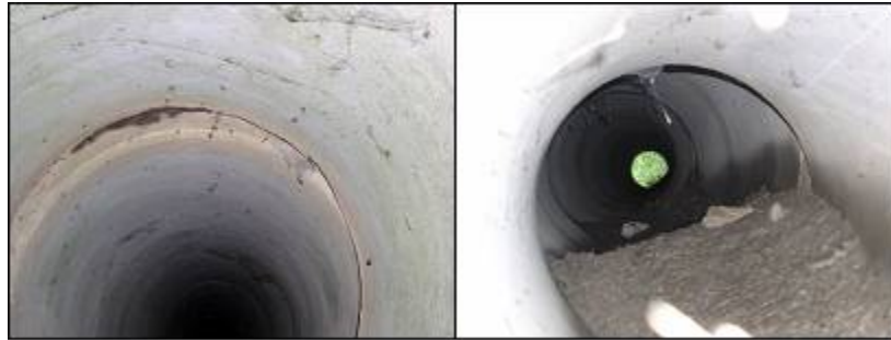
Figure 2.3 Culvert Pipe showing Cracks and Joint Separation (Najafi et. al 2008)
