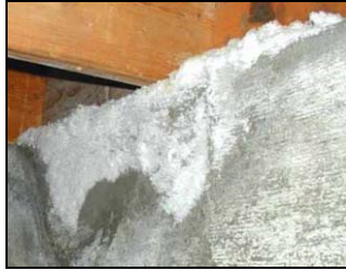
Figure 2.9 Formation of Efflorescence on a Concrete Surface.
