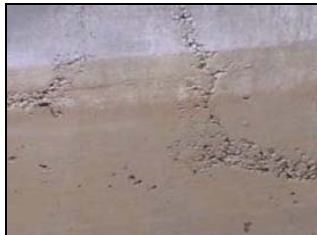
Figure 2.10 Honeycombing on a concrete surface.
