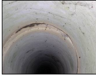
Figure 2.5 Transverse Cracks in a Culvert Pipe (Najafi et. al. 2008)
