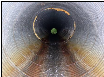
Figure 2.1 Corrosion in Culverts (Najafi et. al. 2008)
