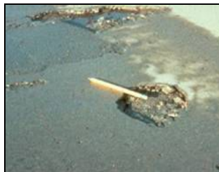
Figure 2.8 Spalling on a Concrete Surface.
