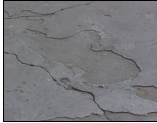
Figure 2.7 Delamination on a Concrete Surface.
