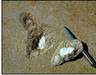
Figure 2.11 Pop-outs in a Concrete Structure.
