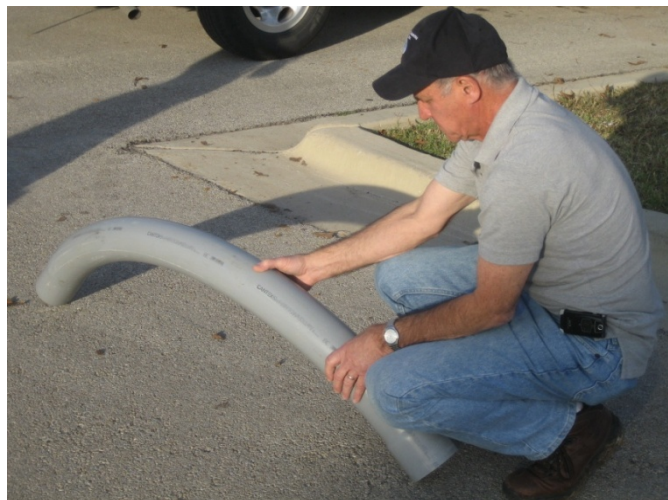
Figure 4-24 PVC Bended Pipe to Join the Two Main Installations
